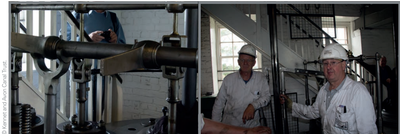
Throttle arm breakage on the Boulton & Watt No.1 engine Crofton Pumping Station, July 2017. This occurred early in the start process and no further damage was caused to the engine. A temporary repair was made to enable operation to be resumed, pending professional conservation advice on permanent repair. This incident was an opportunity to review and improve inspection, maintenance operational and safety procedures, along with conservation and recording practices.
