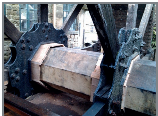
Restoration work in progress on a waterwheel from Abbeydale Industrial Hamlet, a unique example of an 18th and 19th Century water-powered industrial works on the River Sheaf in Sheffield. By 2004, both the tilt wheel shaft and the grinding hull wheel shaft had been repaired numerous times, and they were too rotten to support the weight of the wheels in rotation. New shafts were sourced from tree trunks of the correct diameter. Due to the scheduled ancient monument status of the site and Grade I listed buildings, the rotten shafts had to be moved out of their wheels without using any part of the building to lift from. Each of the shafts weighed between 2 and 3 tonnes with their cast iron ends fitted.
